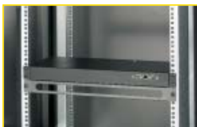
Rack concentrator (for communication of the signals from the sensors to the computer network)
